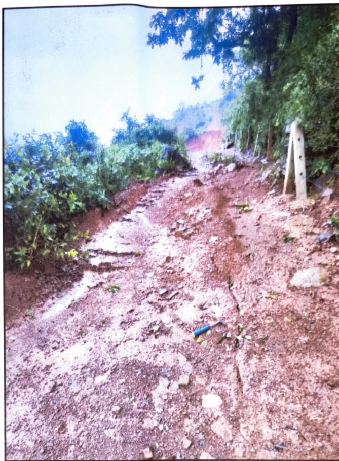
Fig. 6 Transverse cracks on the left flank of the landslide
